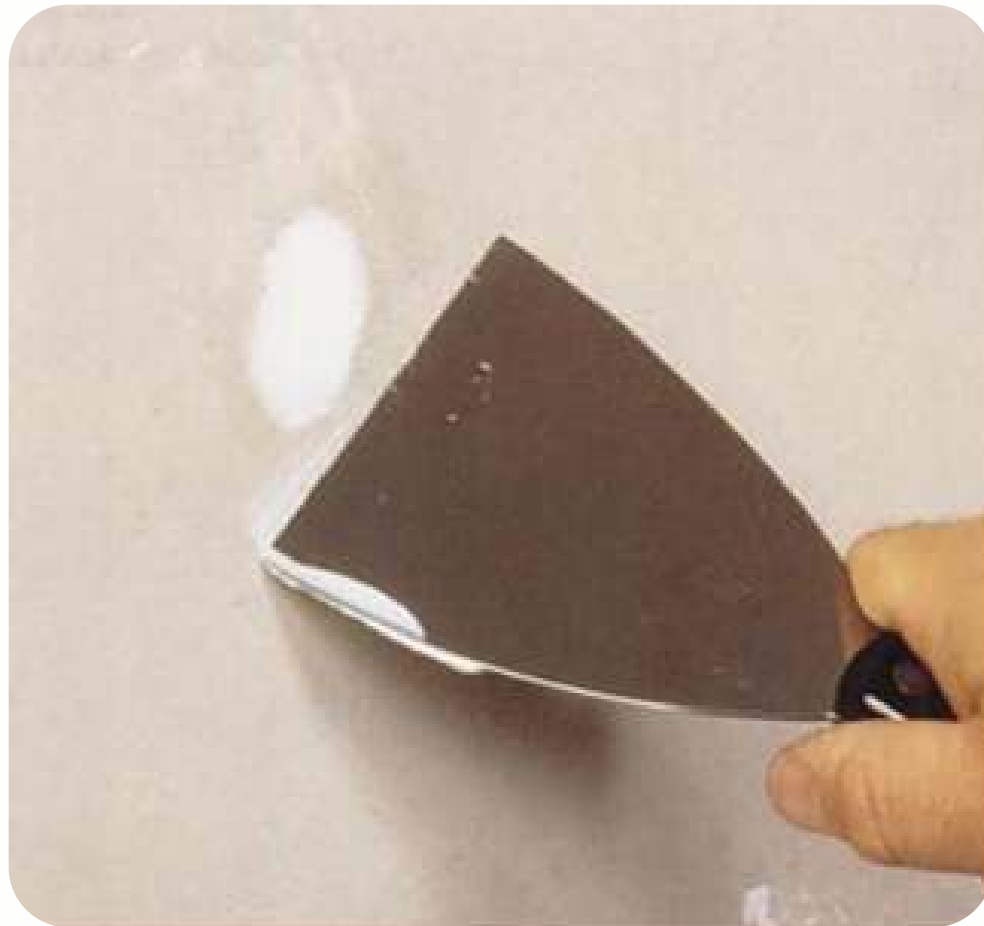
Pinholes and Hairline Cracks
